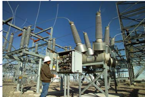
Power Grid Test Bed
